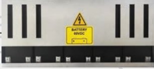
Akü Grubu Batteries For Emergency
